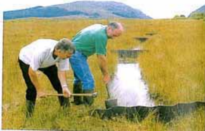
Drain blocking, Croaghonagh, Co. Donegal
