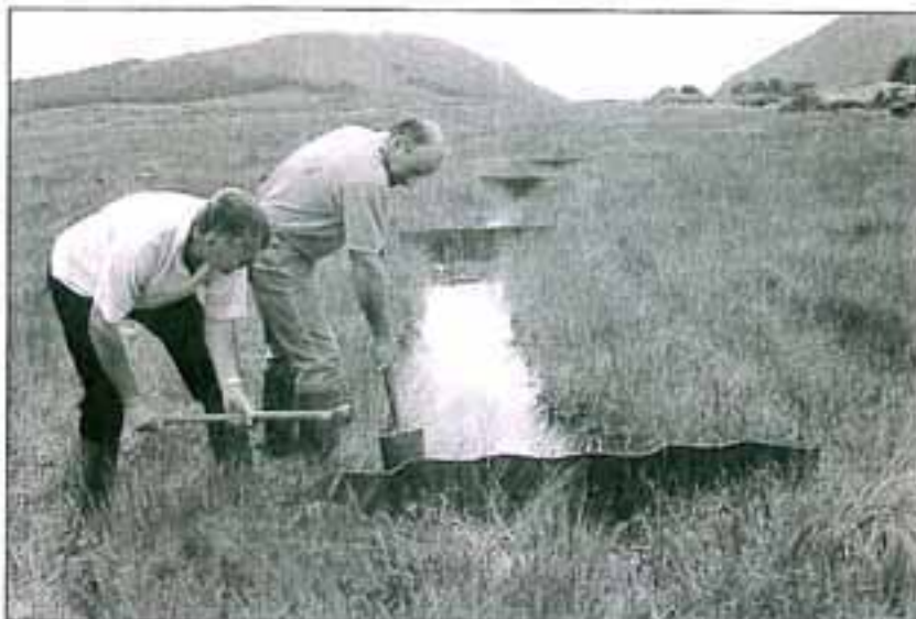
Drain blocking at LIFE Site, Croaghonagh, County Donegal
