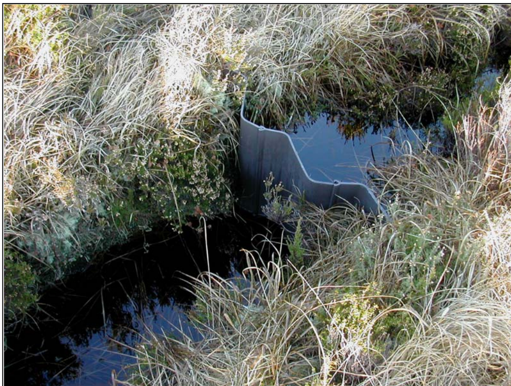
A view of a plastic dam in a drain at the site. Note that the water level is higher on the right hand side of the dam which shows that water is being retained. Photograph taken in August 2007.
